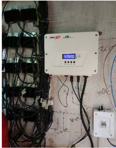
Figure 10 The optimizers and inverter
